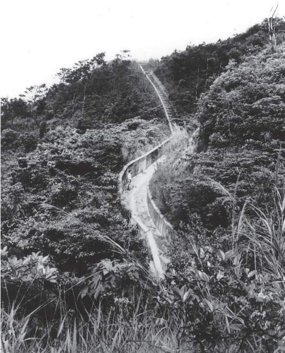
Figure 18. Reinforced concrete rock trap ditch below Beacon Hill
