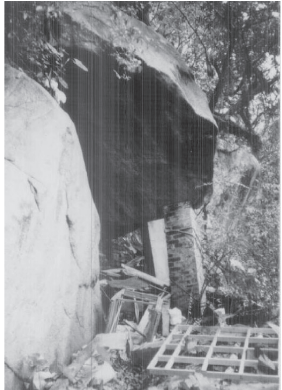
Figure 1. Boulder supported by old brickwork columns
